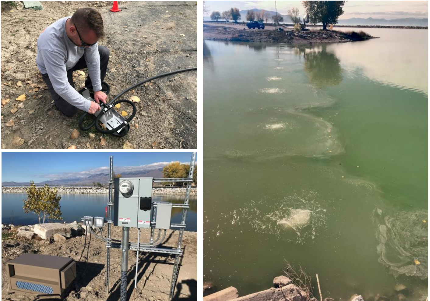
Figure 8: Installation and operational photos of bubble curtain at Utah Lake State Park preventing a surge of cyanobacteria from entering the inner marina area from the outer marina.
